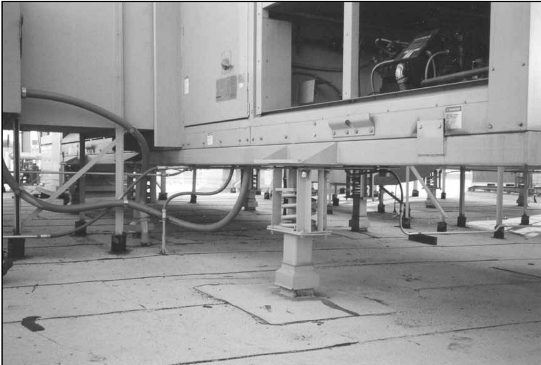
Kinetics FLSS rooftop isolation on a building in Culver City within one mile of the I-10 collapse.
