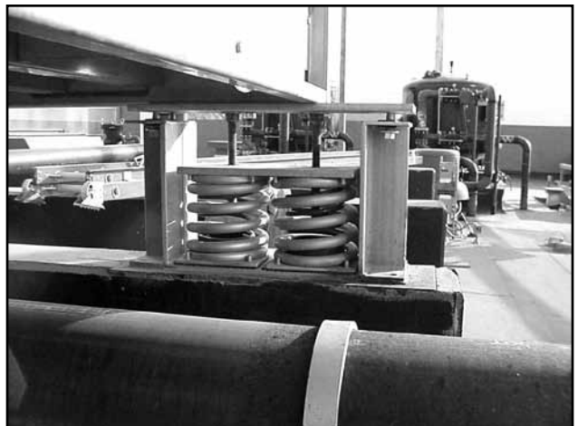
Vertically restrained Spring Isolators used with a cooling tower Fig. 9
