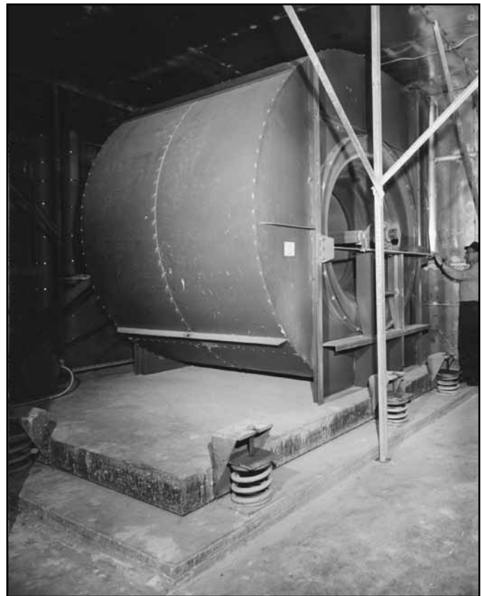
Supply Fan supported by Spring Isolators Fig. 4
